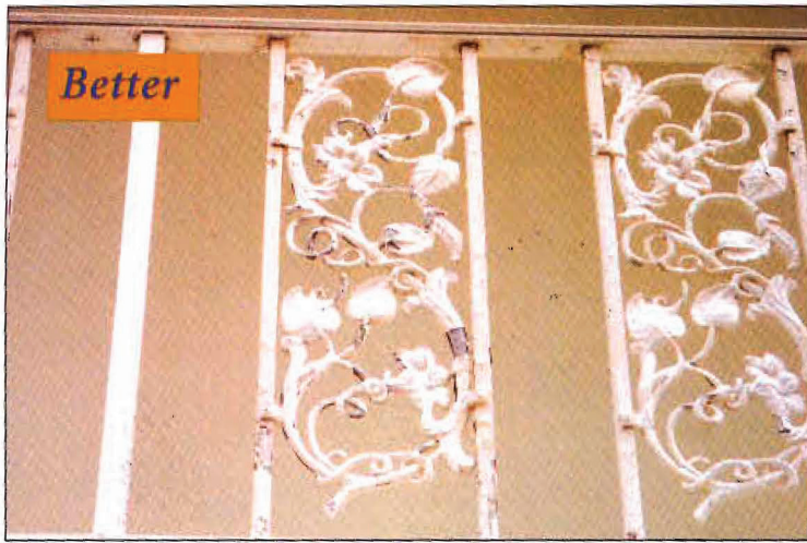
This flower panel in West Palm Beach, FL, shows flaking because of a poor coating job. But its marine grade castings are still shiny and coherent after eight years.
