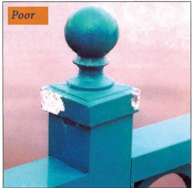
This 2" ball cap is not marine grade. It shows chalk corrosion and flaking (starting at corners) after four years on the Indian River in Vero Beach, FL.
